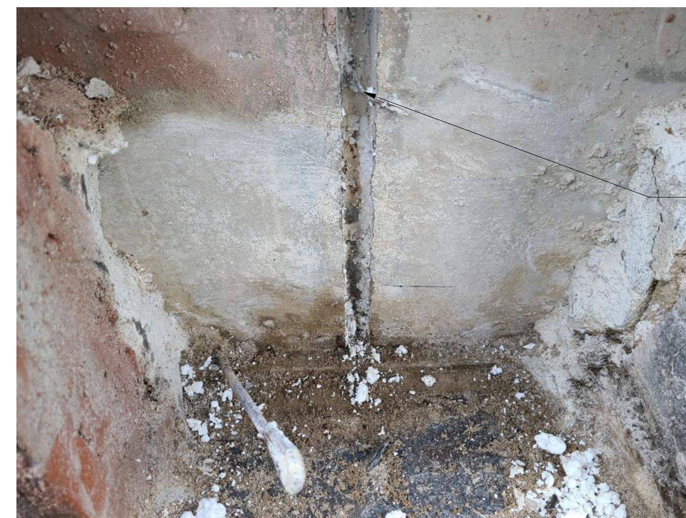
10 PHOTO OF DOVETAIL SLOT IN BACKUP WALL AT TEST CUT SCALE: NONE
