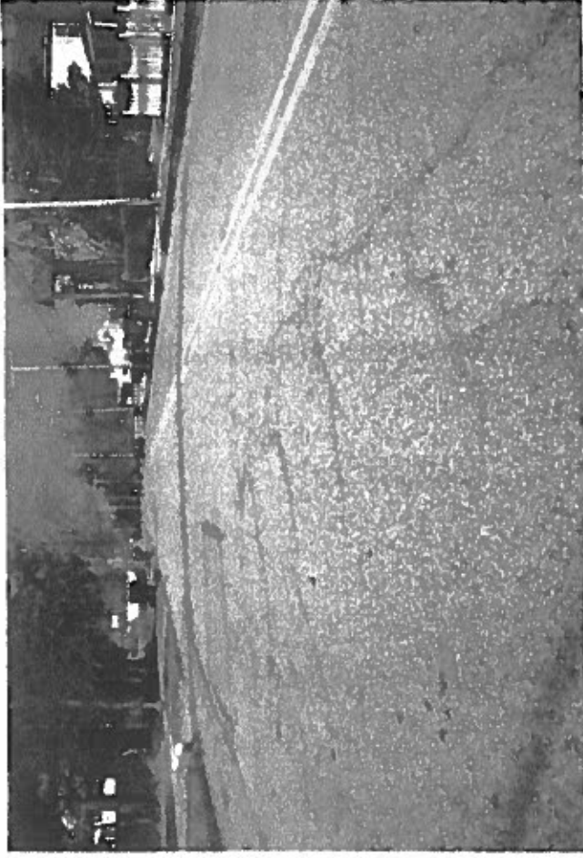
Cracks in Pavement #2
